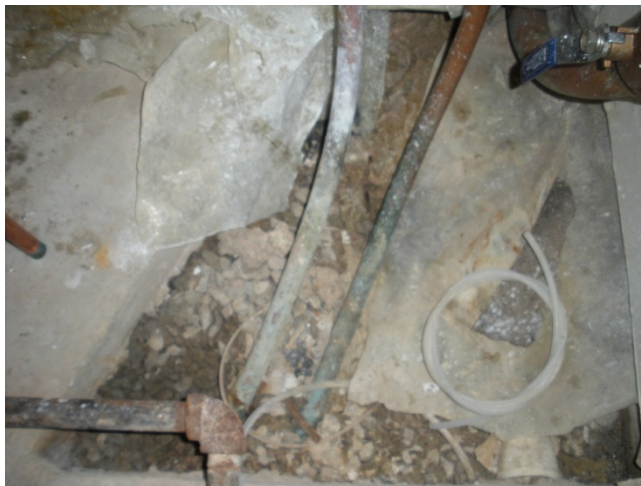
Corroded copper pipes below the main water meter on the east side of the basement.
